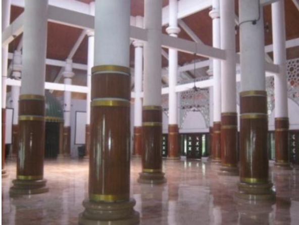
Figure 5. The new construction of the Ampel Mosque Building with reinforced concrete frames
