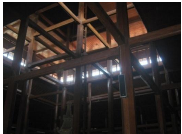
Figure 4. The original construction of the Ampel mosque building with teak wood frame
