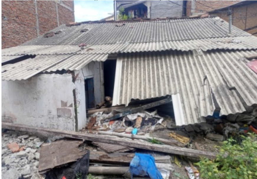
Figure 2. Damage to several building structures is the impact of the position of the land surface
