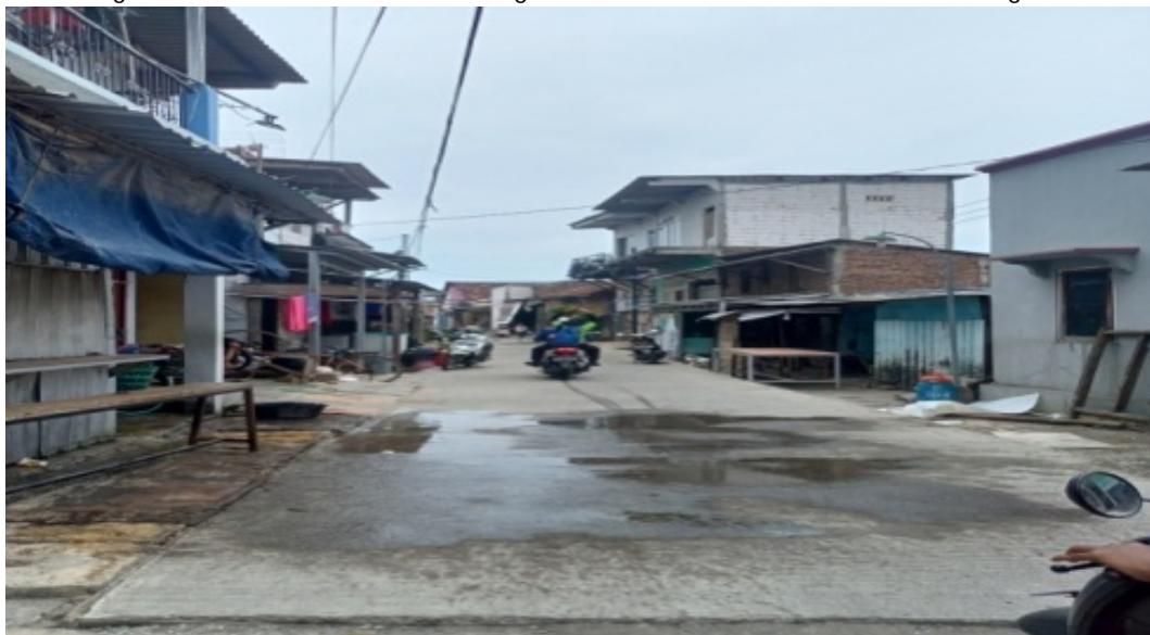
Figure 4. Road elevation is also being carried out so that seawater does not stagnate
